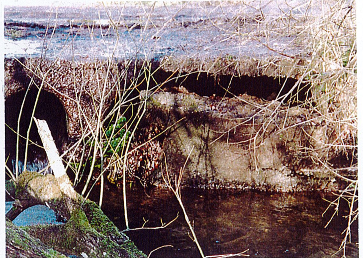
KNACKERS HOLE COLLAPSED CULVERT
